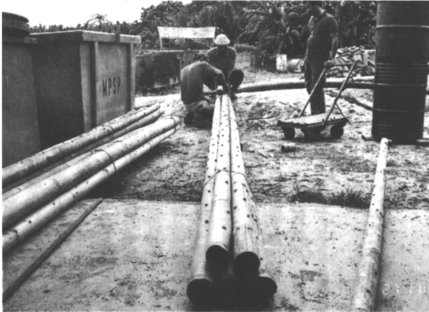
Picture 3.2 Leachate collection pipes made of bamboos (From Dr. Matsufuji. Fukuoka Univ. "Semi Aerobic Landfill Site Story" "Mizu" Jan & Feb 1998.)
