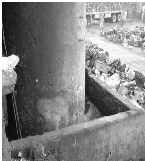
Filthy Condition of Emission Treatment Unit
